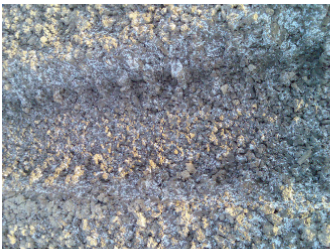
Figure 2. Aerated G1 emulsion mix showing evidence of salt crystallization appearing overnight.
