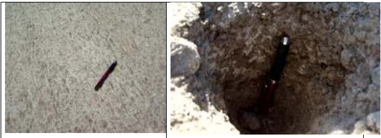
Figure 1. Salt dust on trial section of G1 base surface and density hole soon after construction.
